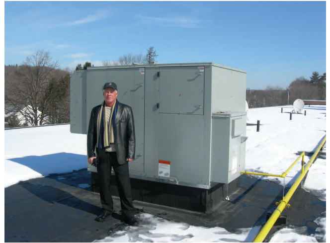
Installation Contractor Dan McCabe standing next to new ERV with Airxchange wheels installed at Doherty Memorial High School.
