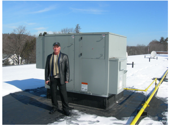
Installation Contractor Dan McCabe standing next to new ERV with Airxchange wheels installed at Doherty Memorial High School.
