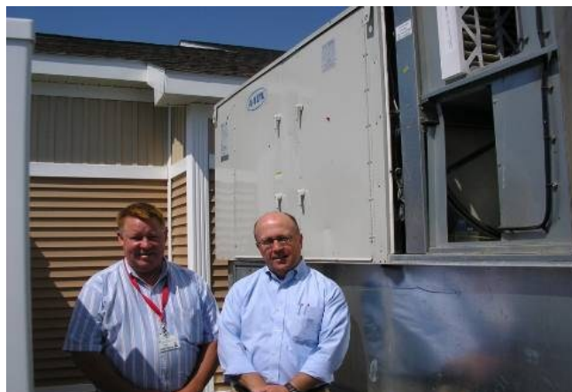
Tom Gray, Director of Facilities Management for Northeast Health (left), and Russ Bailey, P.E., of SMRT.
