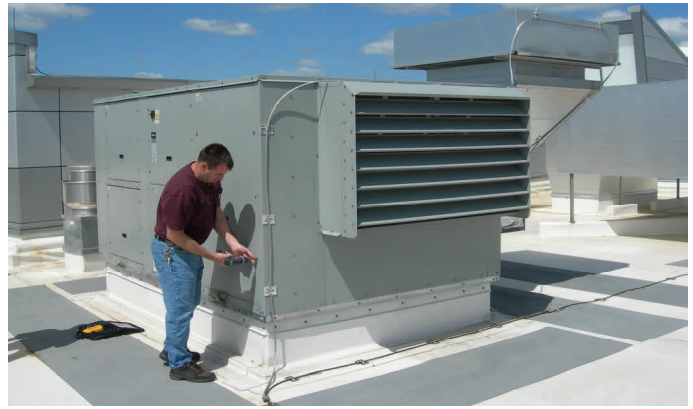
HVAC Technician Brian Polak preparing to check an energy recovery wheel for cleanliness.
