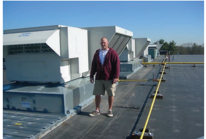
Custodian Tim Fournier comments there is no added maintenance for the energy recovery wheels.
