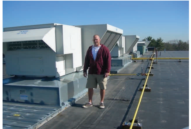
Custodian Tim Fournier comments there is no added maintenance for the energy recovery wheels.
