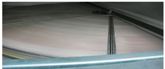
Installed in the school's rooftop HVAC unit, the Airxchange ERV wheel dramatically reduces the cost of conditioning outside air (OA) by recovering and recycling energy from exhaust air, significantly reducing the OA (and total) load on the HVAC system.
