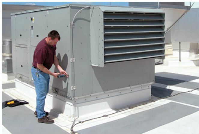
HVAC technician Brian Polak is impressed with how the energy recovery wheels keep PCTA in the comfort zone.
