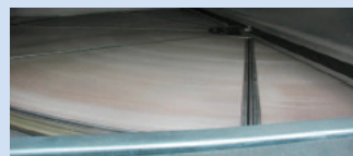
Installed in the school's rooftop HVAC unit, the Airxchange ERV wheel dramatically reduces the cost of conditioning outside air (OA) by recovering and recycling energy from exhaust air, significantly reducing the OA (and total) load on the HVAC system.
