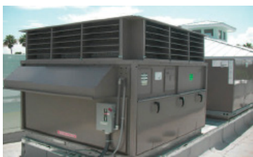
Because ERVs reduce the outside air load on the HVAC system, the rooftop unit at Turtle River is about half the size it would have been without an Airxchange wheel.
